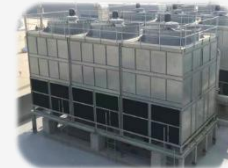
[Out Air Control Unit, QAC]
